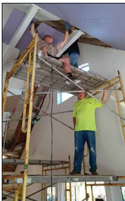
Disaster Relief Ministry volunteers repair a ceiling in Little Gasparilla, Florida in October.
